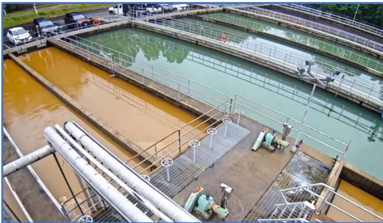
South Rivanna Water Treatment Plant
